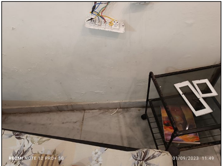
Moisture was noted on back wall
