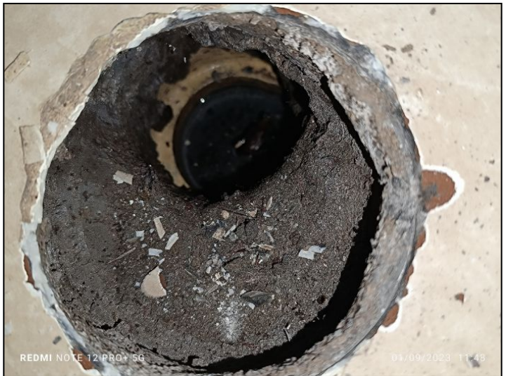
Improper installation of drain pipe
