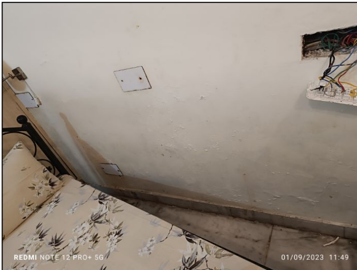
Moisture was noted on left wall
