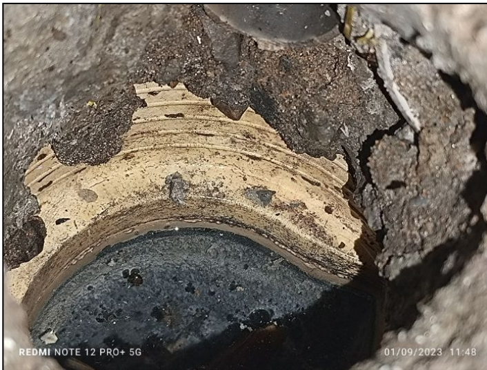
PVC Sleeve was not installed inside the drain
