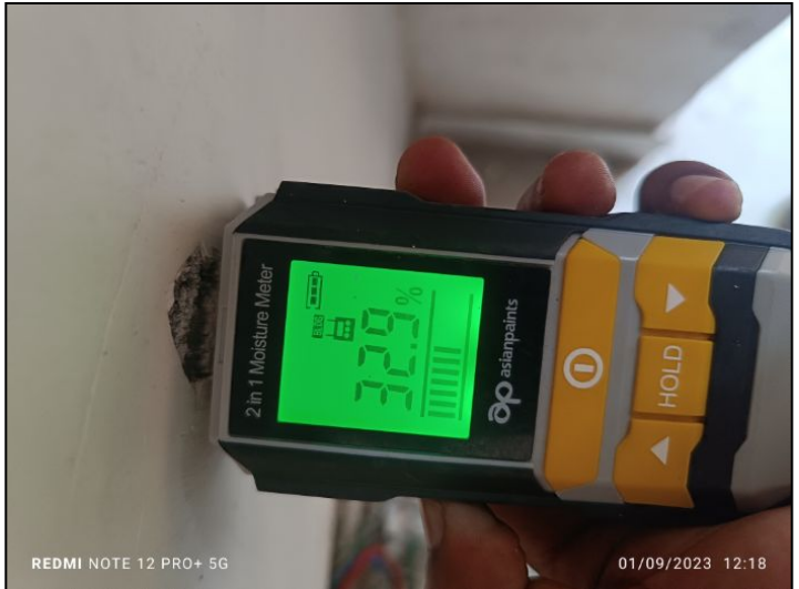
High moisture was noted on office fornt wall
