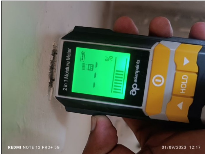
High moisture was noted on office front wall
