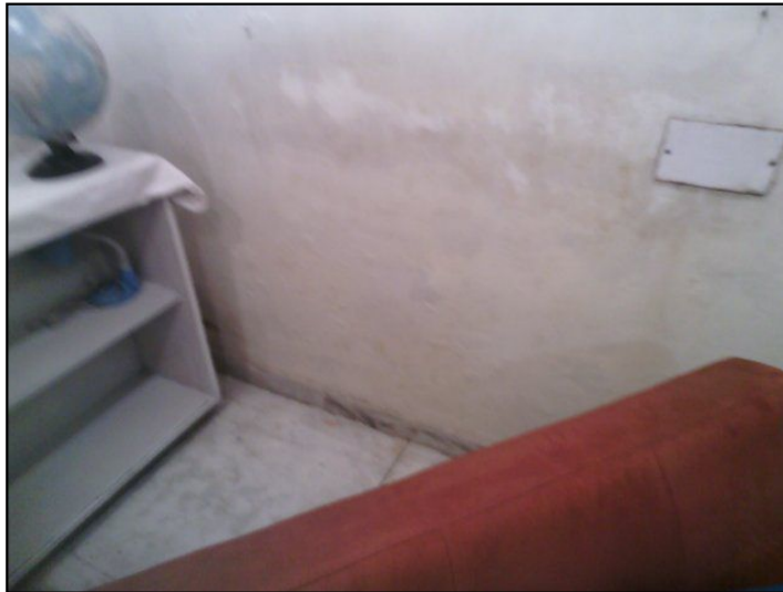
Visual image of moisture on office inside front wall
